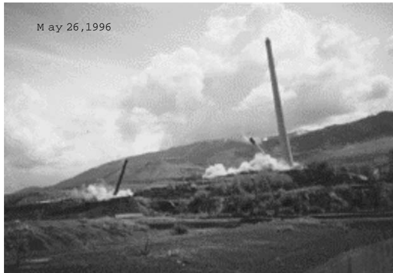
Fig. 1 Demolition of Bunker Hill Mine smoke stacks by U.S. Army Corps of Engineers. A symbolic reminder of the decline of U.S. mining industry.
